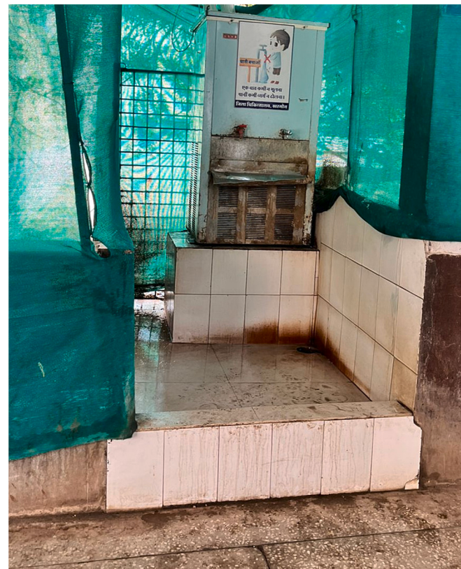
Image 13. Drinking water facility. An external drinking water facility is seen with obstructions such as thresholds. The floor is seen to be wet.
